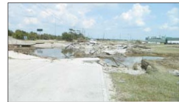
The San Jacinto River washed out Market Street, taking a new path.
