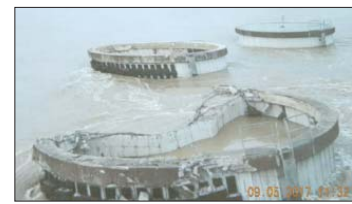
Bumpers meant to protect the I-10 bridge were damaged by Harvey.
