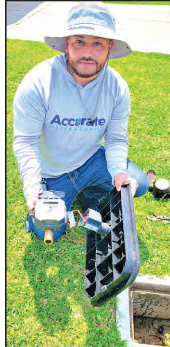
Francisco Hernandez of Accurate Metering LLC is installing the Badger meter with BEACON transmitter and antenna to North Channel Star writer Allan Jamail's water line. (Photo by Allan Jamail)
