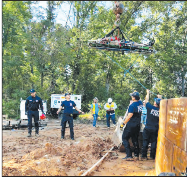
The 100-foot structure where the contractor fell is located close to Westlake Houston Parkway and North Lake Houston Parkway. It is the site where they were laying new water lines from the City of Houston water treatment plant near Lake Houston.
