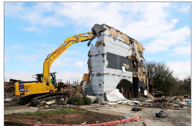
Demolition began shortly after the political figures left the property which was the site of at least nine fires over the last year.
